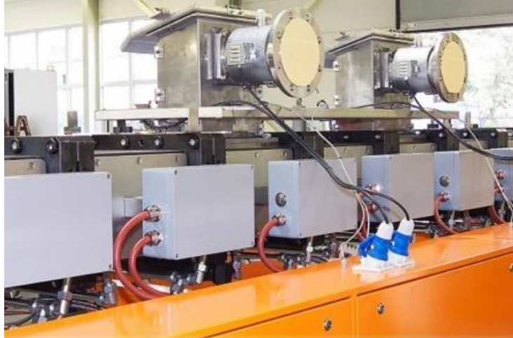
Heated vent stacks equipped for vacuum hook-up on ZSE-MAXX process section
